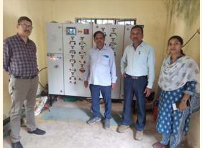
Process Control Panel
