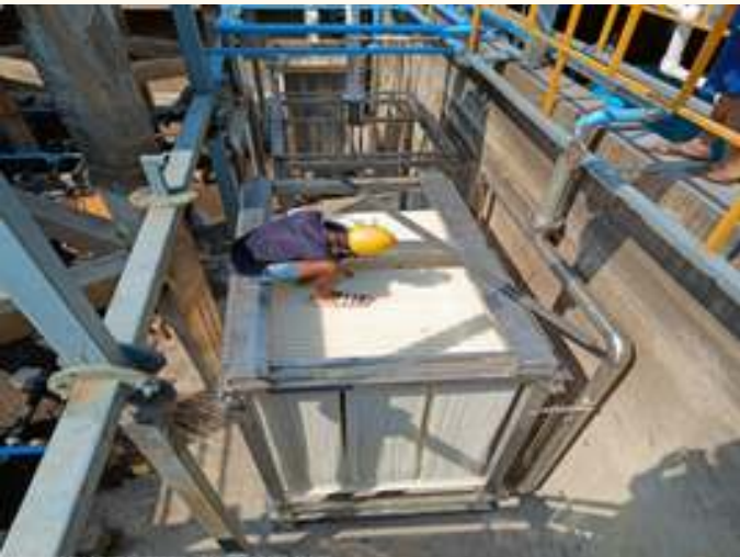
Membrane Bio Reactor set up
