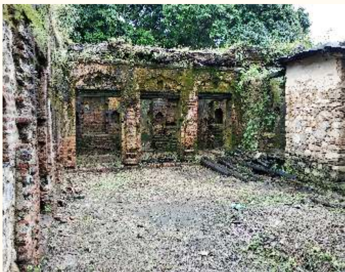
A view of the old dilapidated structure
