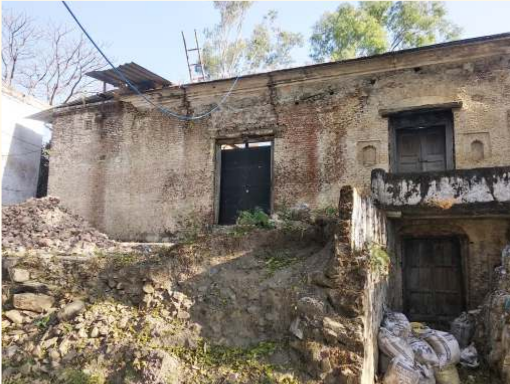
Old Dilapidated Structure before implementation of the project
