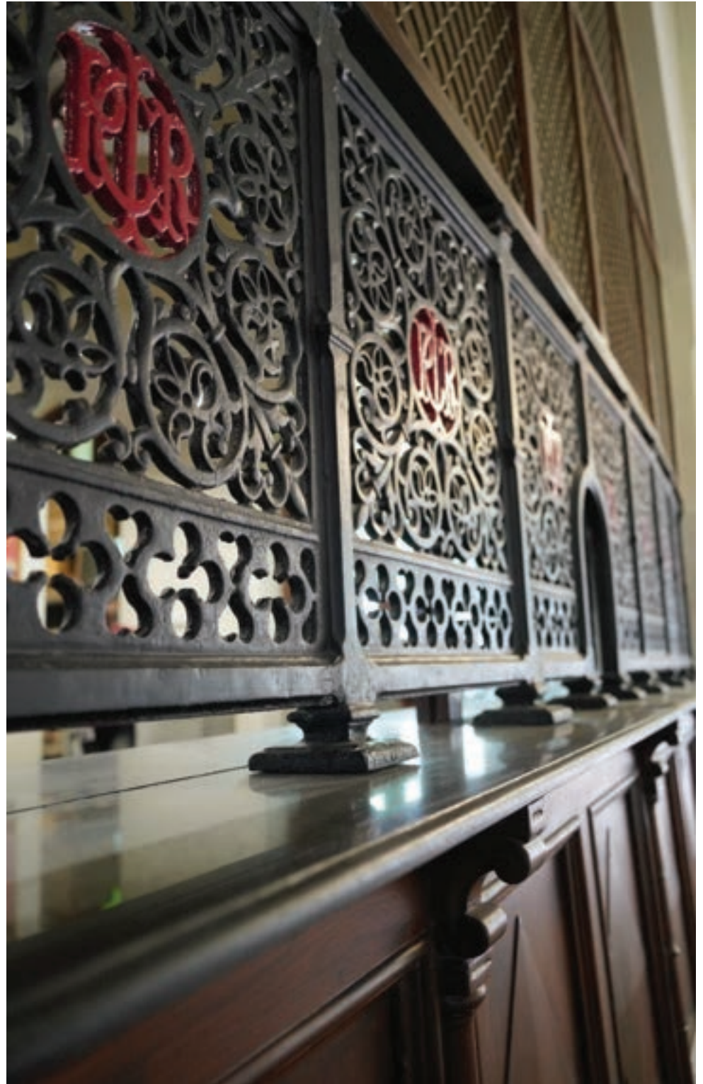
Restored original cast iron grill with the initials GIPR (Great Indian Peninsula railway).
