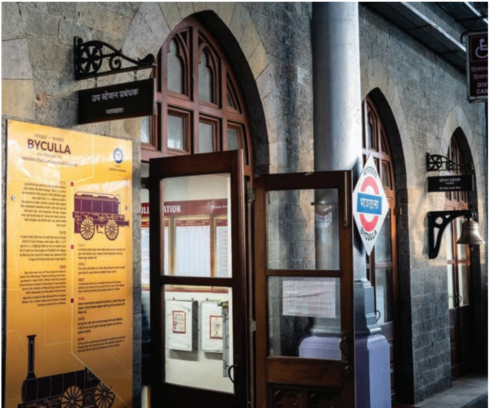
Exposed basalt concourse façade with restored teal wood doors and cast iron bracket signage.
