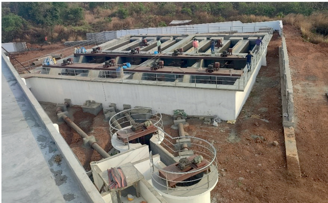
Water Treatment Plant at Kondotty Municipality, Kerala
